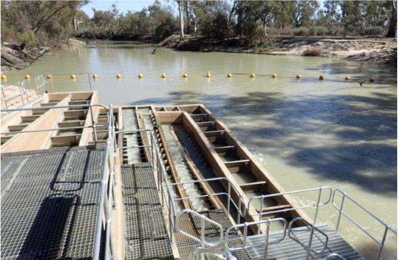
Photo 2 – Fishway downstream of Pipeclay Weir at Chowilla. Photo: SA Water
