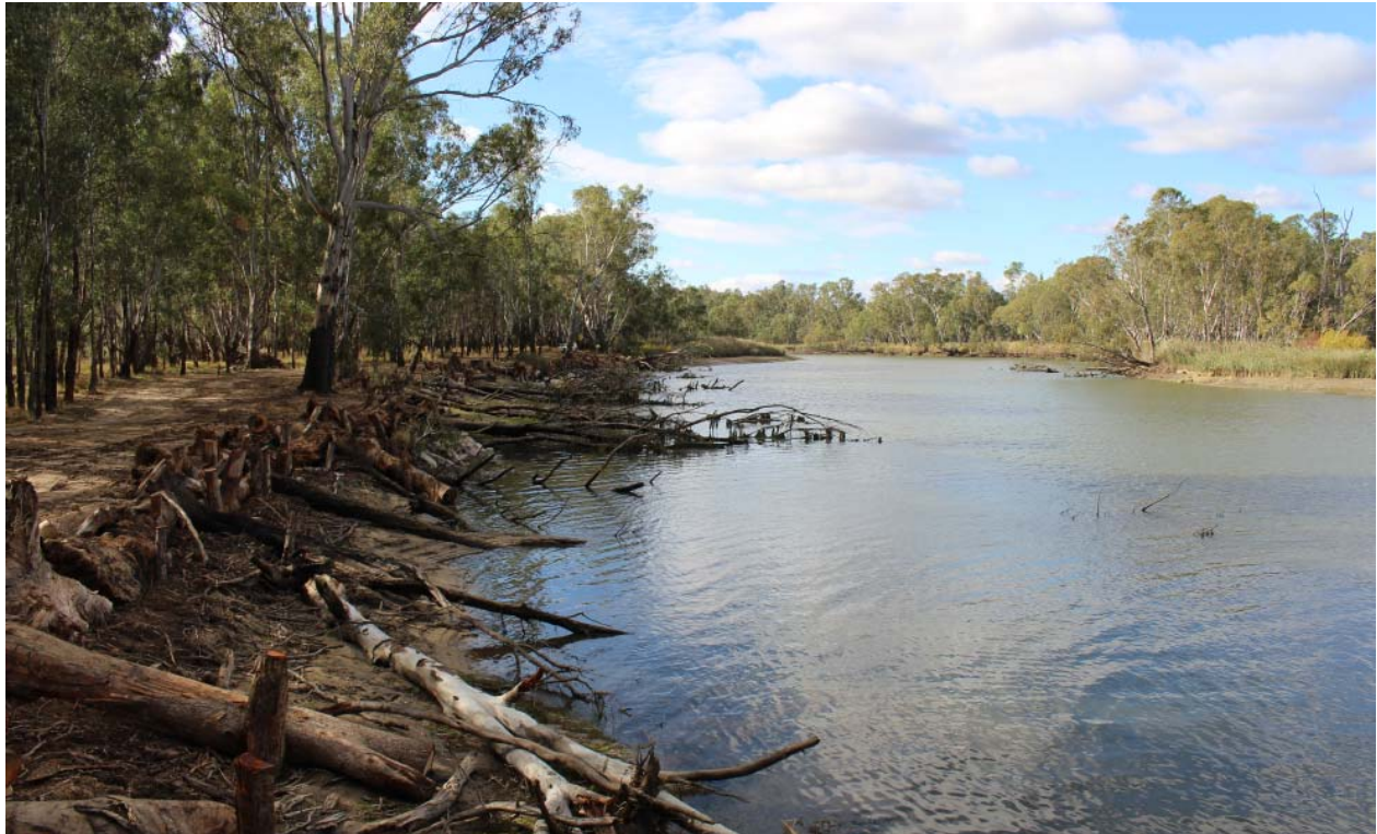
Photo 1 – Recently completed erosion protection works on the River Murray just upstream of Bundalong (photo courtesy Hugo Bowman, MDBA)
