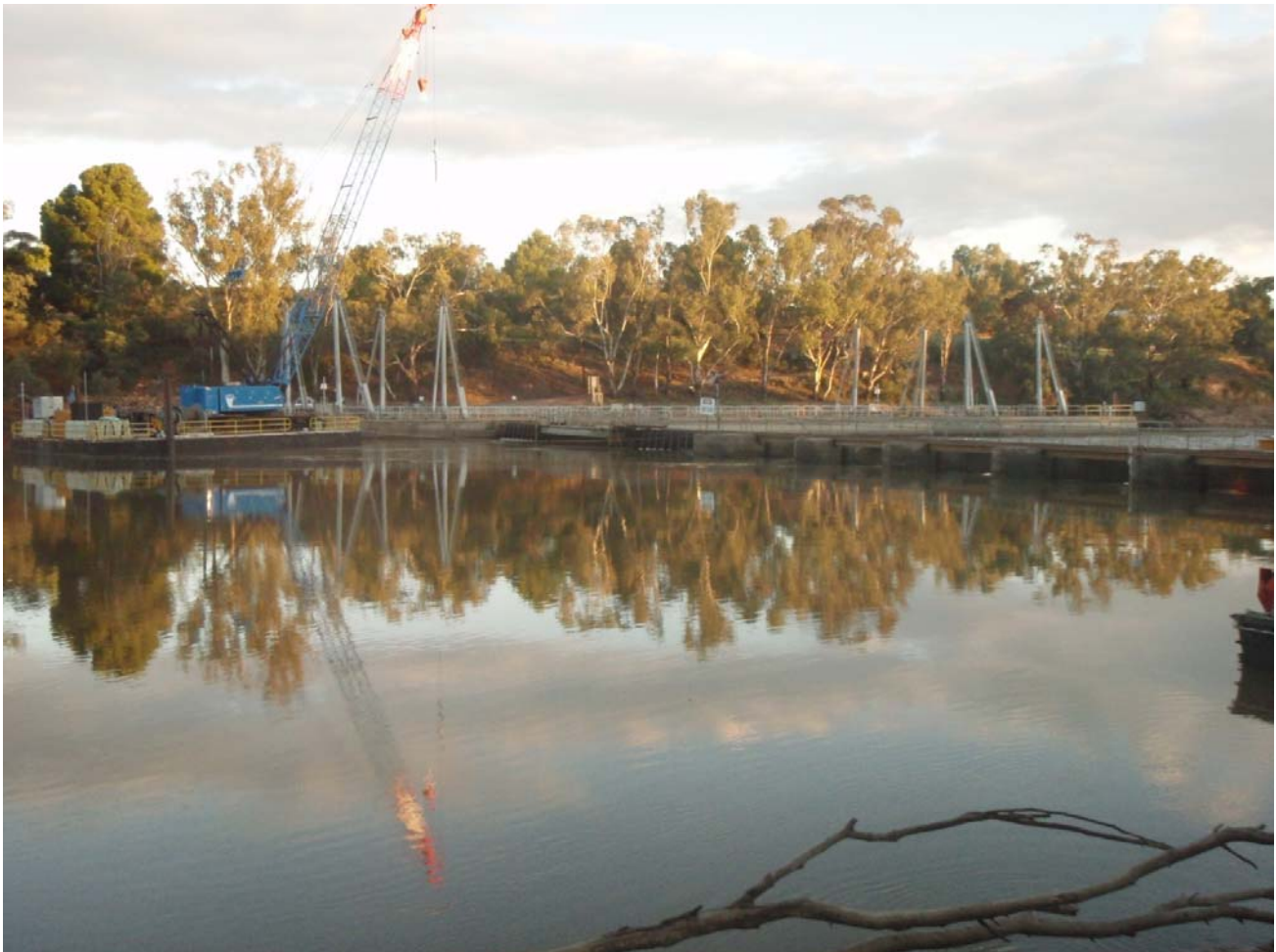
Figure 1– Euston Weir was re-instated during the week and construction work on the new navigable pass has re-commenced (Photo: John Prentice, MDBA ).
